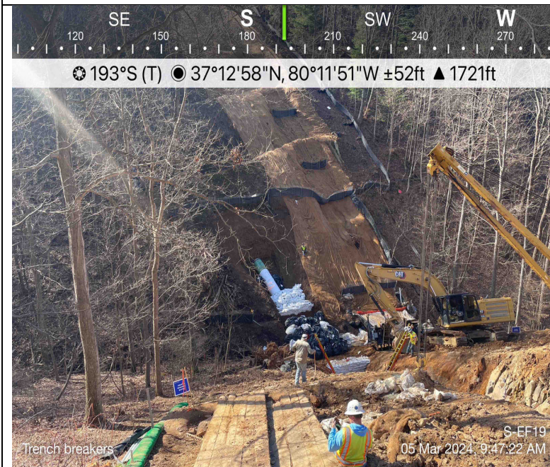
Photo Description: Trench breakers for G.A.S. & C.I.S installed prior to backfill of pipe.
