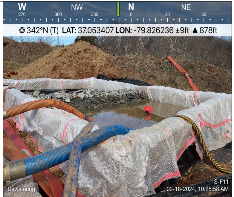
Photo Description: An overview of one of the the dewatering structures used on-site during the crossing.
