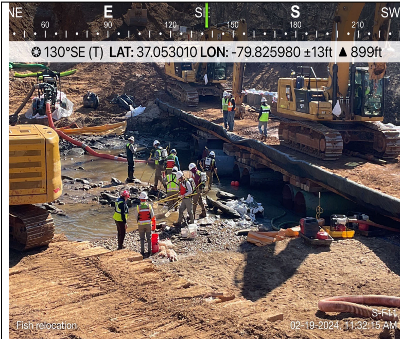
Photo Description: The fish relocation was conducted after installation of the dam and pump around.
