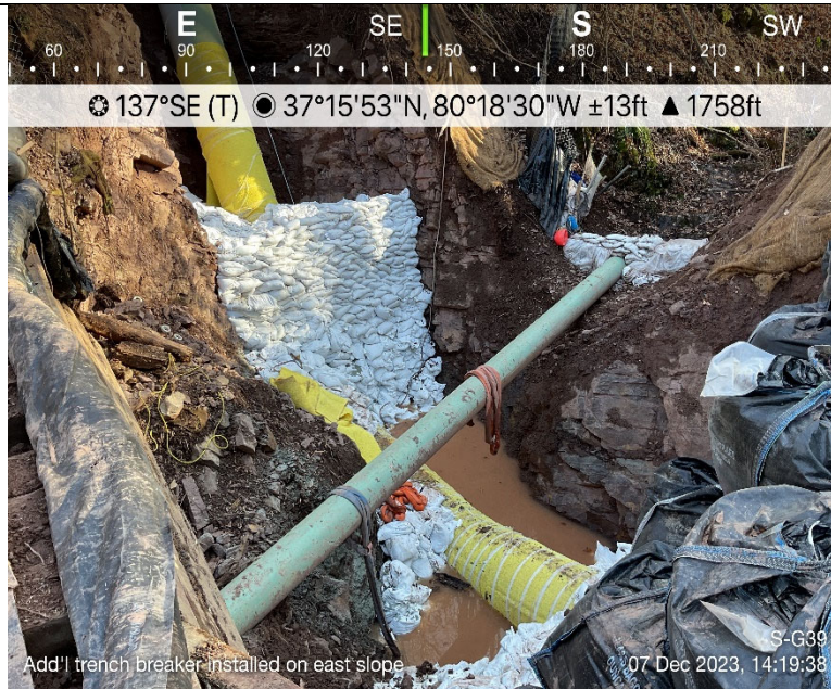
Photo Description: Pipe lowered into trench and beginning of sandbag backfilling on GAS of resource. Resource flumed throughout crossing activities.
