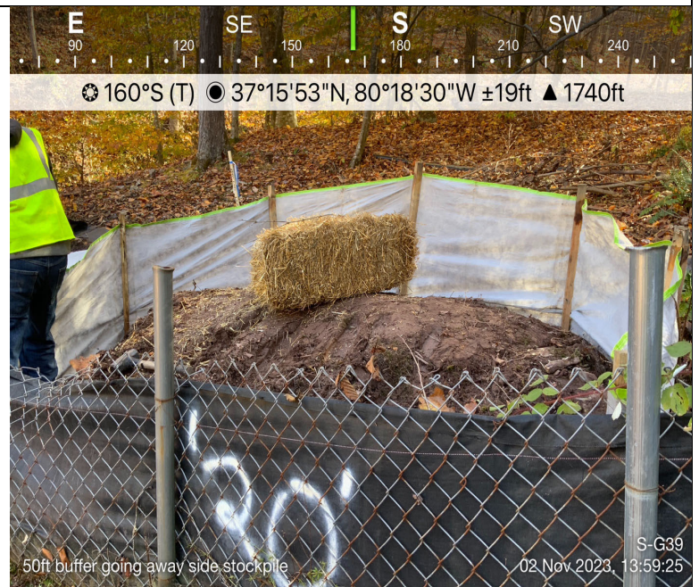
Photo Description: Top soil stockpile on the going away side of the pipe.
