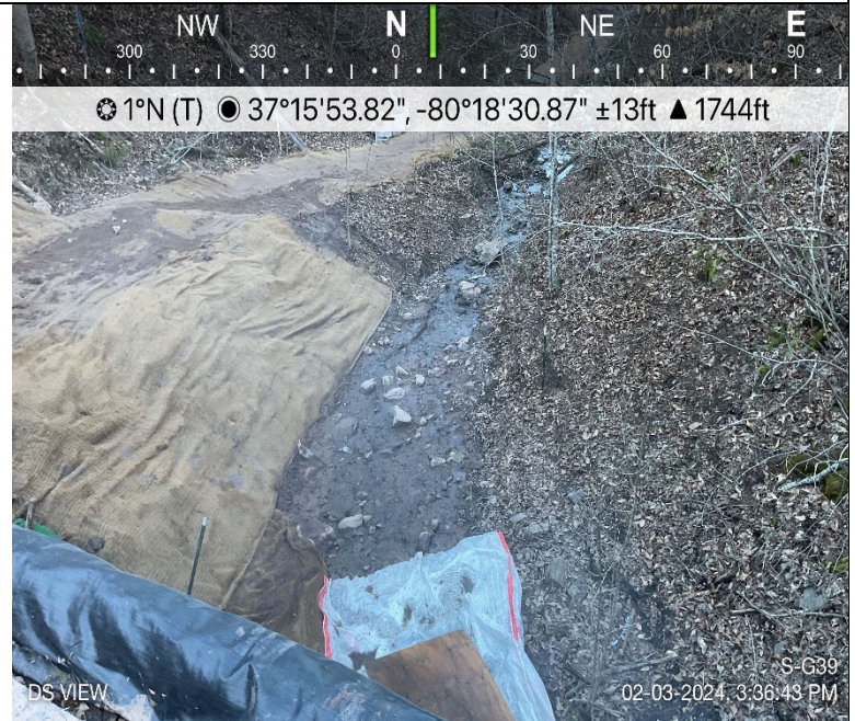
Photo Description: Areas impacted for the remediation effort were seeded and stabilized with erosion control matting.
