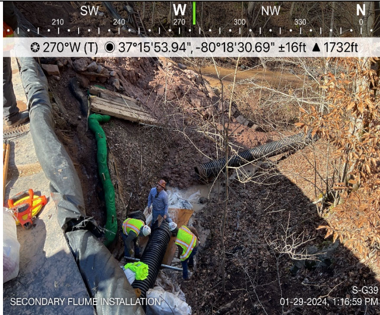
Photo Description: Secondary flume installation to extend flume past the area needed to be disturbed for remediation.
