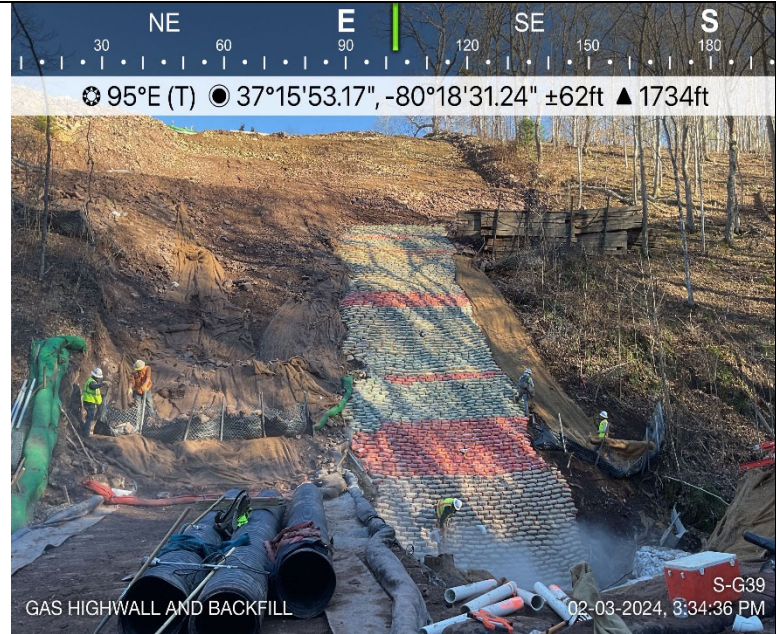
Photo Description: Highwall construction was completed on the GAS of the resource. MVP Specification MVP-44A, 44B, & 45.
