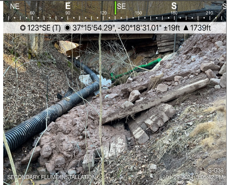
Photo Description: Alternative angle of the right of way slip into the downstream area of S-G39.
