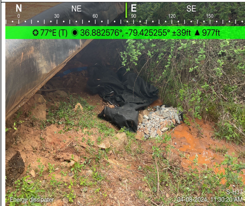
Photo Description: Energy dissipater for dam and pump around.
