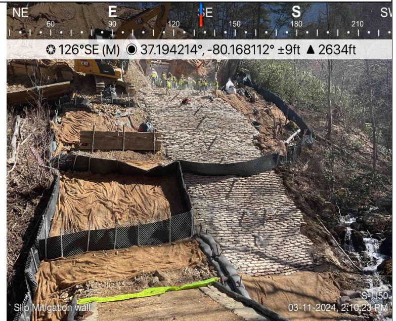
Photo Description: The slip mitigation wall during construction. Wall construction began outside the OHWM of resource.
