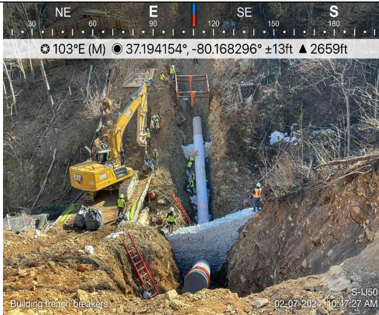
Photo Description: The trench breakers were constructed around the pipe on both the CIS and GAS of the resource.
