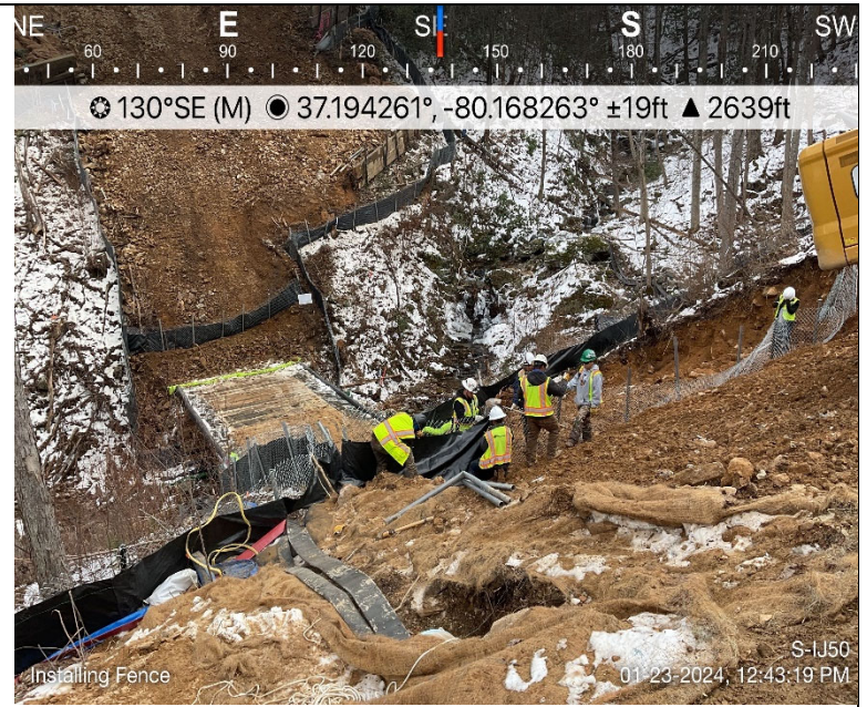
Photo Description: Super silt fence was installed around the workspace and maintained as needed throughout the crossing duration.
